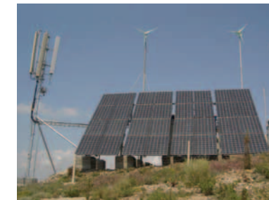
Remote Telecommunication System
