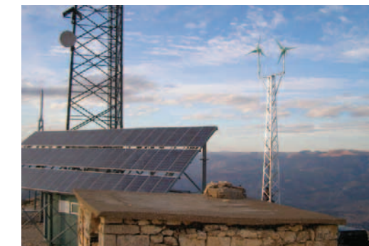
Remote hybrid wind/PV telecommunication system in Turkey
